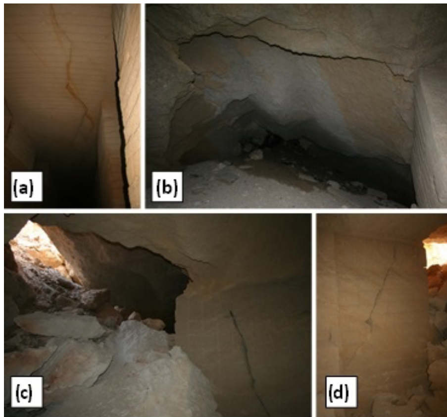
Figure 7. Instability evidence at the Barletta underground quarry: (a) tensile fracturing of the vault; (b) block detachment from the vault; (c) open fractures on pillars, and vault collapses in the area closest to the sinkhole; (d) crushing of pillar with joints (adapted from De Giovanni et al., 2011).
